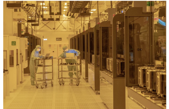
TSMC clean room
